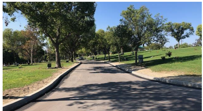
New Concrete Curbs replace the old asphalt curbs around the Park Vista loop.
