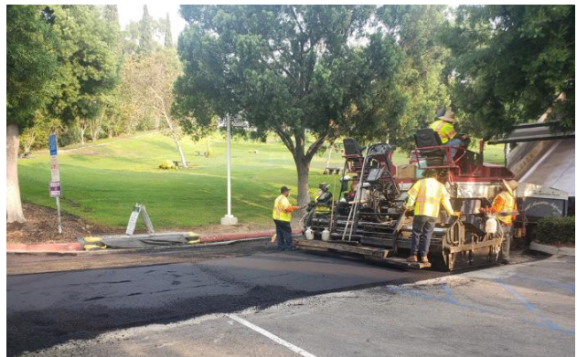
Repaving of the main street from the front gate to the public restroom building.
